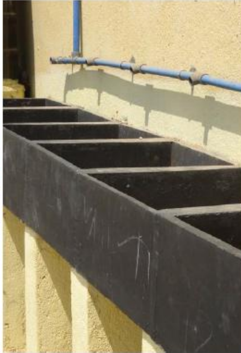
THE WASH AREA WITH NO TAPS
